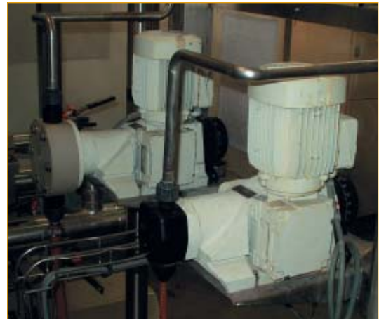
Metering of soda and acid
