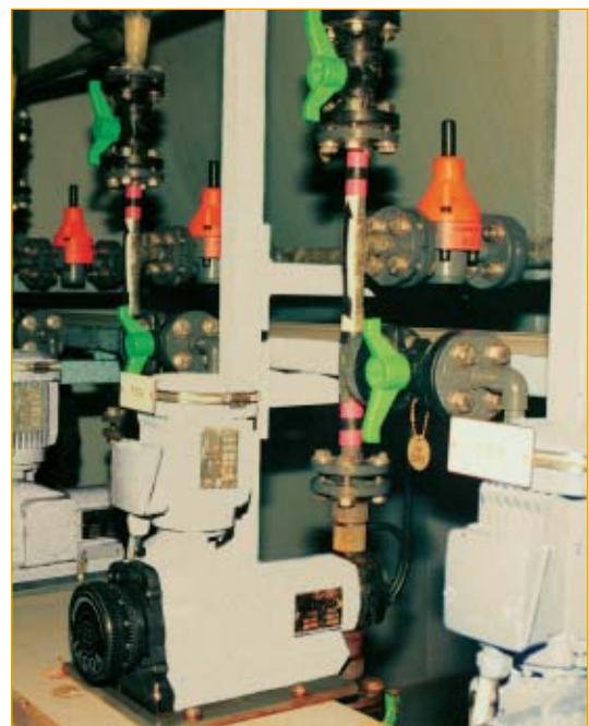
Ferric chloride pumping in purification station
