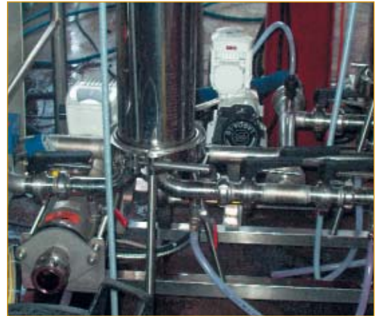
Pump on filtering pallet (wine production)
