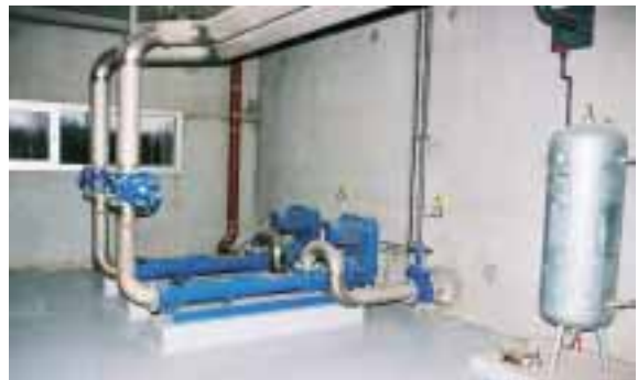
Injection of Polymer (15 bar) proportional to sludge flow
