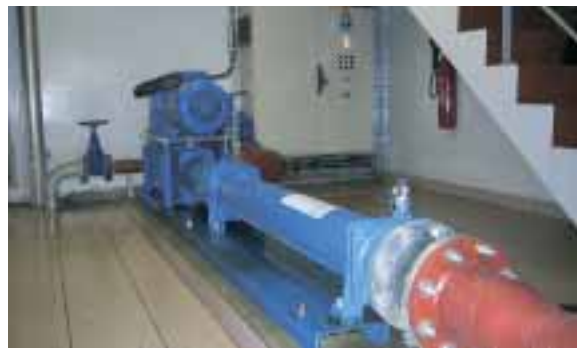
Pump with control box
