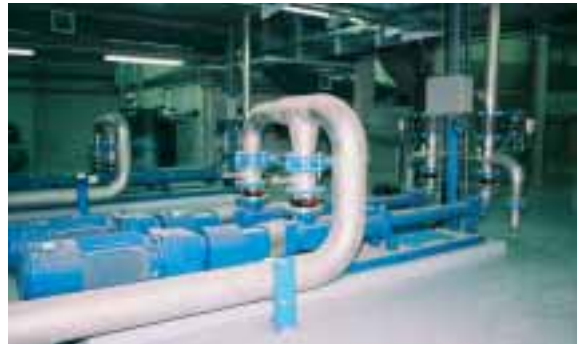
Filter Press Feeding with 2 Moineau Pumps
