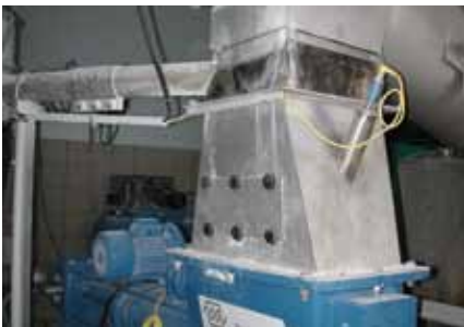
Level control built into a control box.
